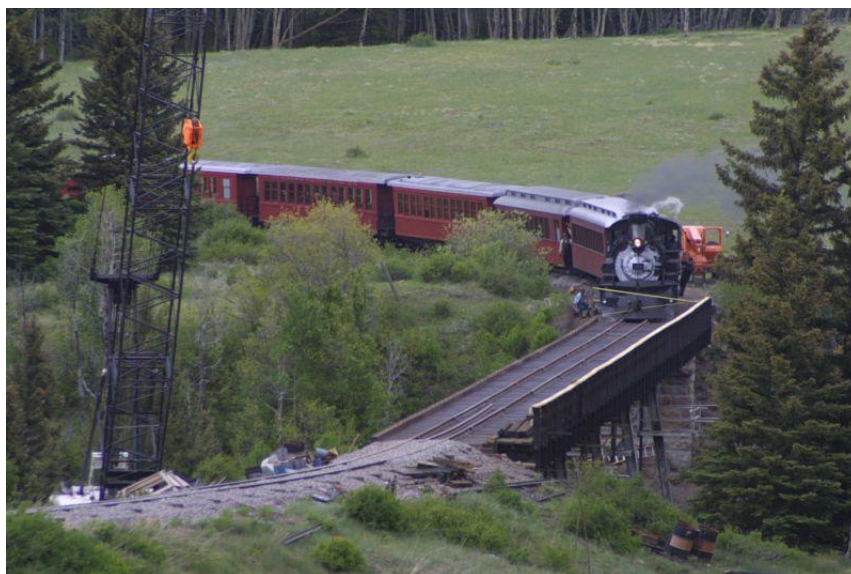
First official train before ripping the ceremonial tape. Lobato Trestle, June 19, 2011. Jay Wimer Photo.
